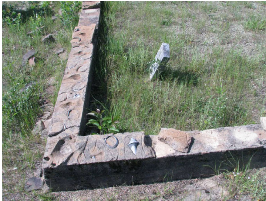
Figure 4. Concrete retaining wall surrounding a family section in Fort Gordon Cemetery 30 (cemetery not included in the geophysical survey).
